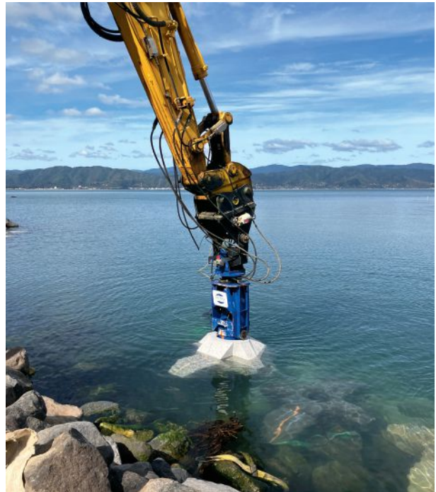
OPERATORS OF EXCAVATORS with grapple attachments needed to move eight different block shapes into place with an 80 mm tolerance.
